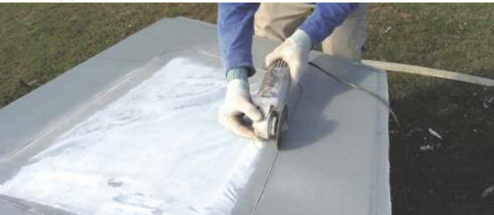
I use a common tile cutting diamond blade on my angle grinder to cut straight lines.
