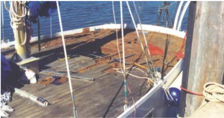
Removing the first bits of teak revealed little steel left, it was now more like soil.
