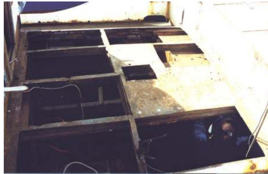
The cockpit was as bad as the aft deck. With so much to replace it was an opportunity to redesign it as well.
