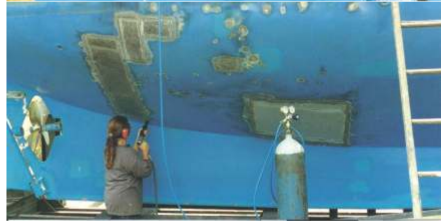
Starboard side patches are in progress at top and above, Kay is using a rattle gun with the scaler tool to chip away any debris and insure the substrate is firm before priming with epoxy.
