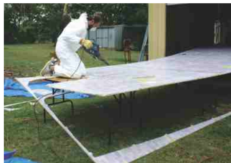
When a bunch of panels are glued together, you just start sawing though some tabs and the sections are released. Clever system!
