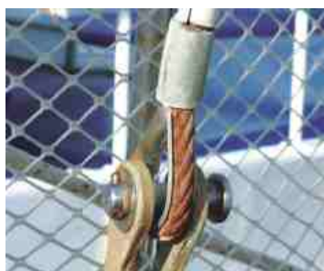
Aluminium swage sleeve, stainless steel thimble and what used to be galvanized wire. The thimble should be gal or solid cast aluminium to avoid galvanic corrosion of the wire.
